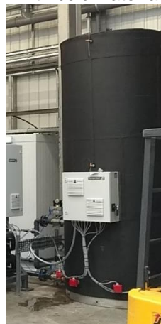
Optional boiler to have pre-heated water
